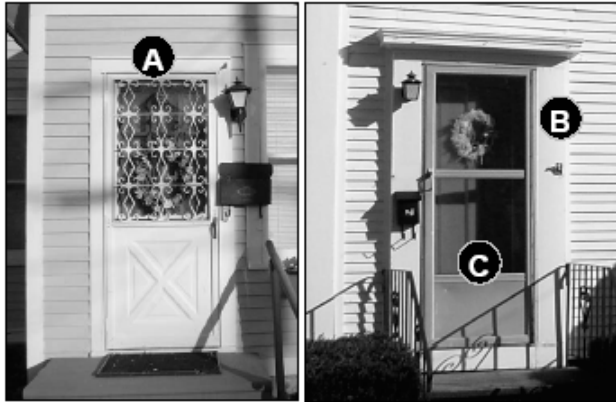
Fig. 22: Examples of improper storm doors. These metal storm doors are mounted on the surface of the wood trim. The white door includes unnecessary detail which does not match the historic design of the house, while the bare aluminum door should be painted.
