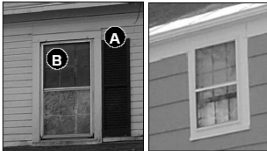
Fig. 24: Examples of improper window treatment. The window on the left has only one (non-functional) shutter, and the storm window is unfinished bare aluminum. The window on the right has a painted storm window, but it is mounted directly to the trim.
